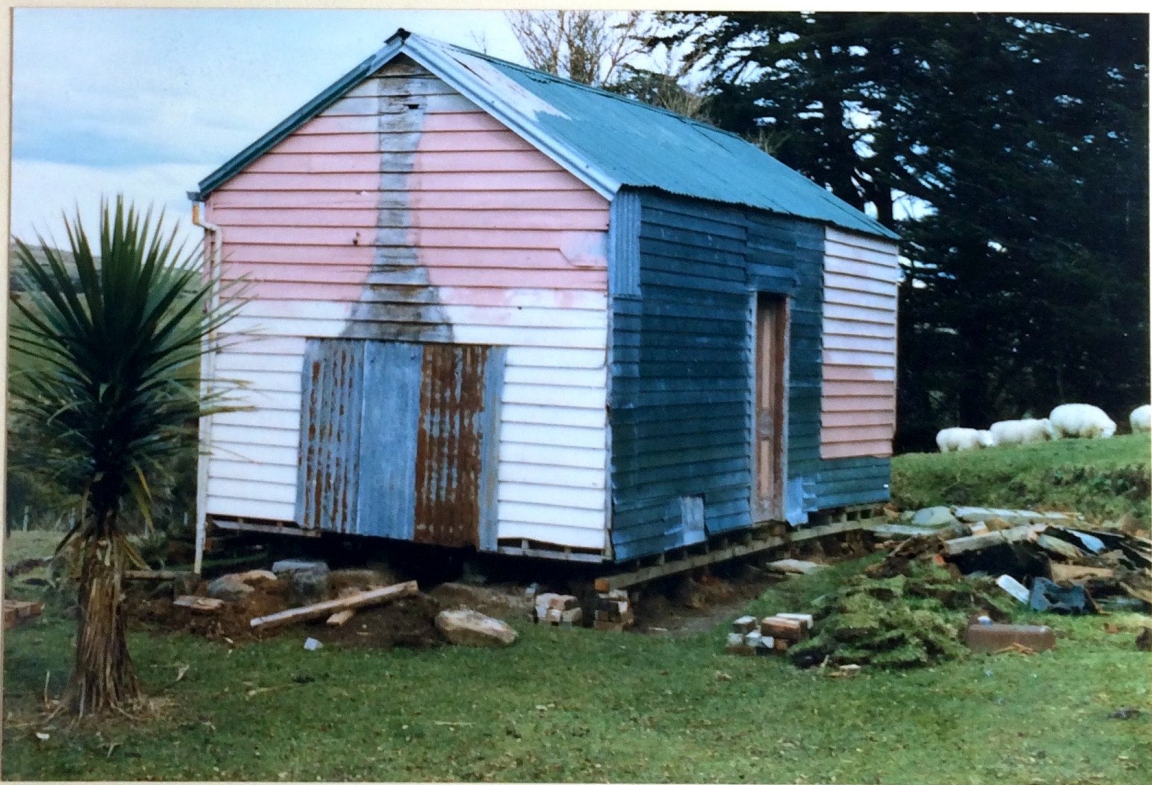
June 1983. The cottage (Rimu Whare) after all the rotting lean-tos and the brick chimney had been removed. The cottage has been weather proofed and some temporary piling done. For several years I tried to get others to commit themselves to refurbishing the cottage. that everybody aged should be saved. My brother Peter and I demolished the deteriorating cottage in June 1988.
